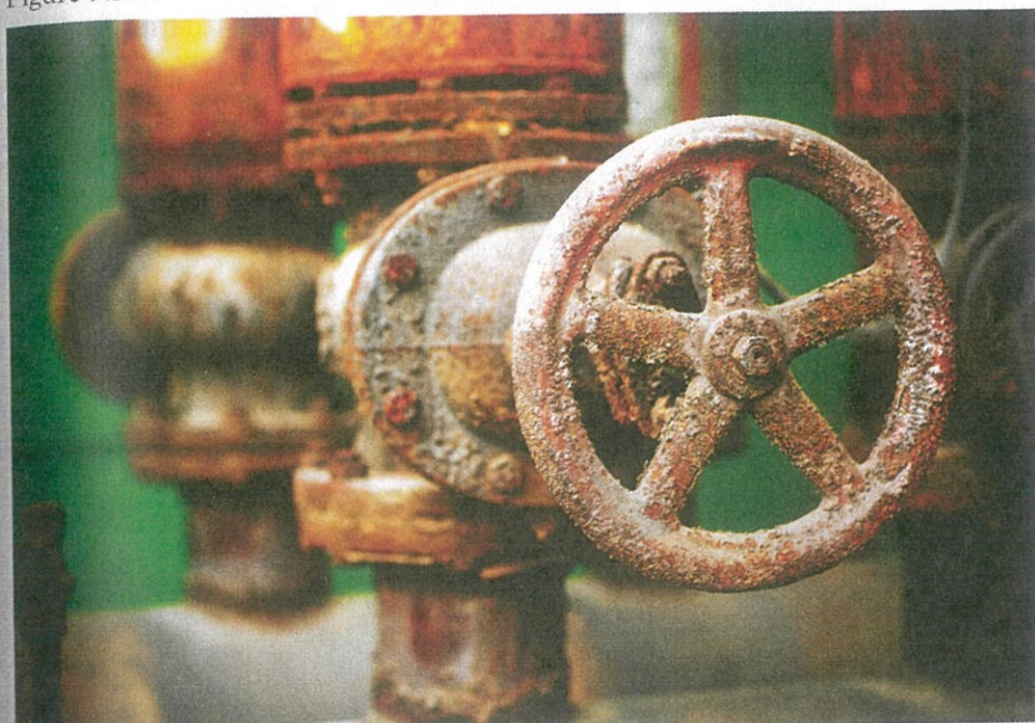
FIGURE 9.5.1 Corrosion is causing water to leak in these pipes in a pumping system.
